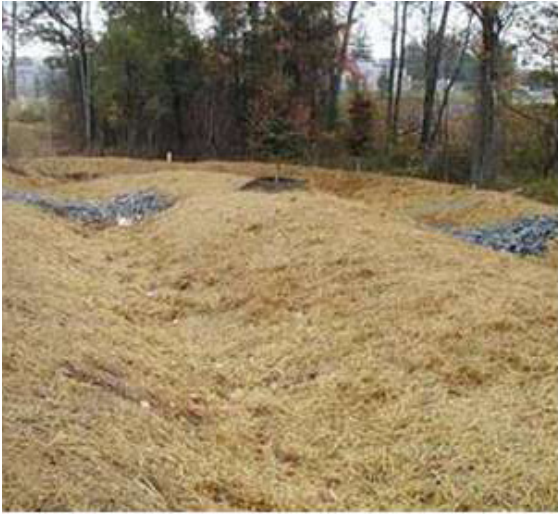
FIGURE 14. Typical dry swale just after construction. (Source: Wetland Studies and Solutions, Inc., Gainesville, VA, 2009.)
