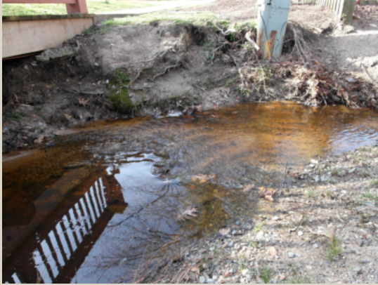
FIGURE 2. Stream channel erosion from stormwater runoff. (Photo courtesy Stephen Mosberg)
