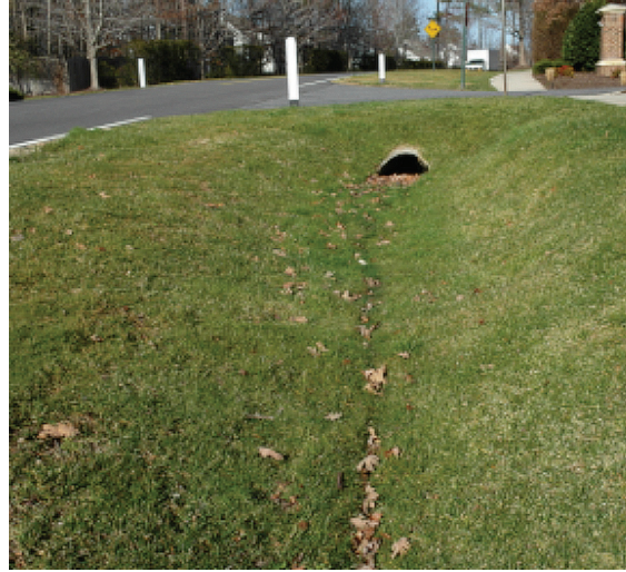
FIGURE 15. An example of a grassed dry swale in a residential application. (Photo courtesy Stephen Mosberg)
